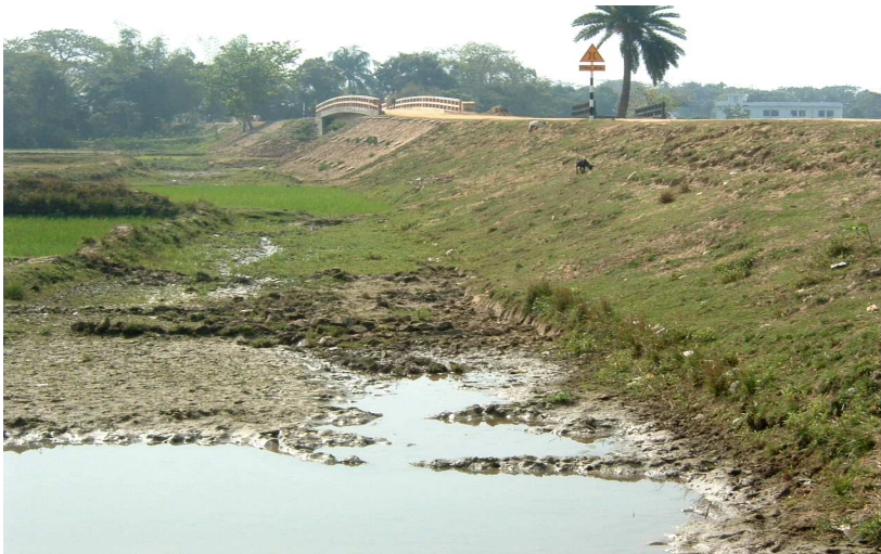
Typical encroachment sapping road banks, with further chance of collapse of the entire structure Photo by Elliott Hurwitz
