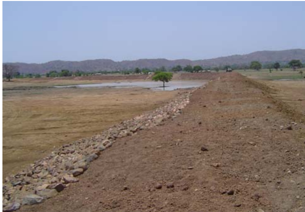
Dam construction at Widnaba (UER). The project has experienced delays in dam construction. Dams are important because, given the low rainfall of the region, no major agriculture intensification is possible without irrigation. IFAD Photo by R.M. Blench.
