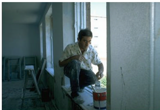
A worker rebuilds a school as part of a community development project
