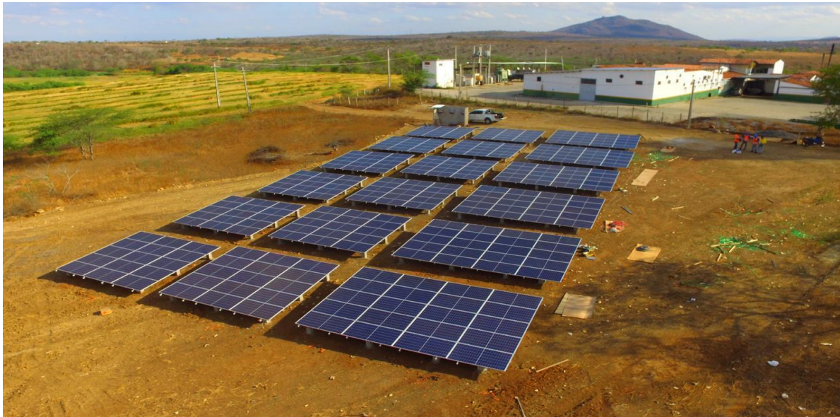
Picture - Solar energy system implemented at COOAPECAL, municipality of Caturité. PROCASE, 2020.
