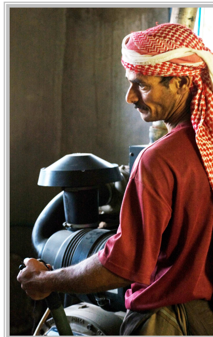
Drinking water pump. The provision of drinking water supply systems was one of the most effective activities financed by the RADP
