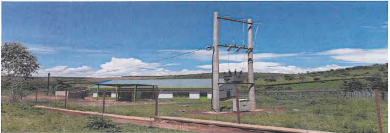
MCC is connected to 3 phase Electricity in Nyagatare district May 2021.
