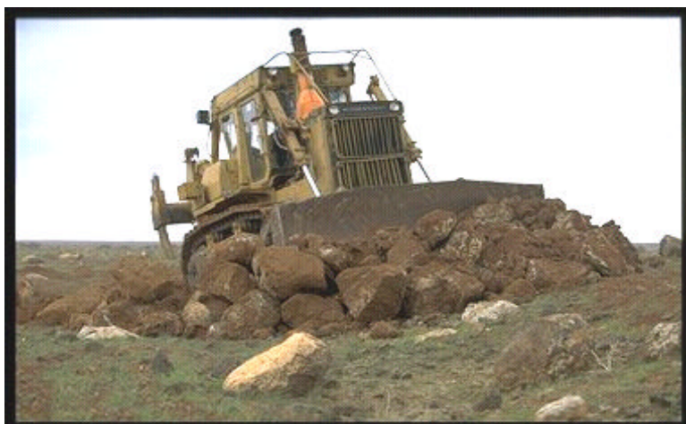
Bulldozers clear fertile land covered with volcanic rock. IFAD photo by Jon Spaul.
